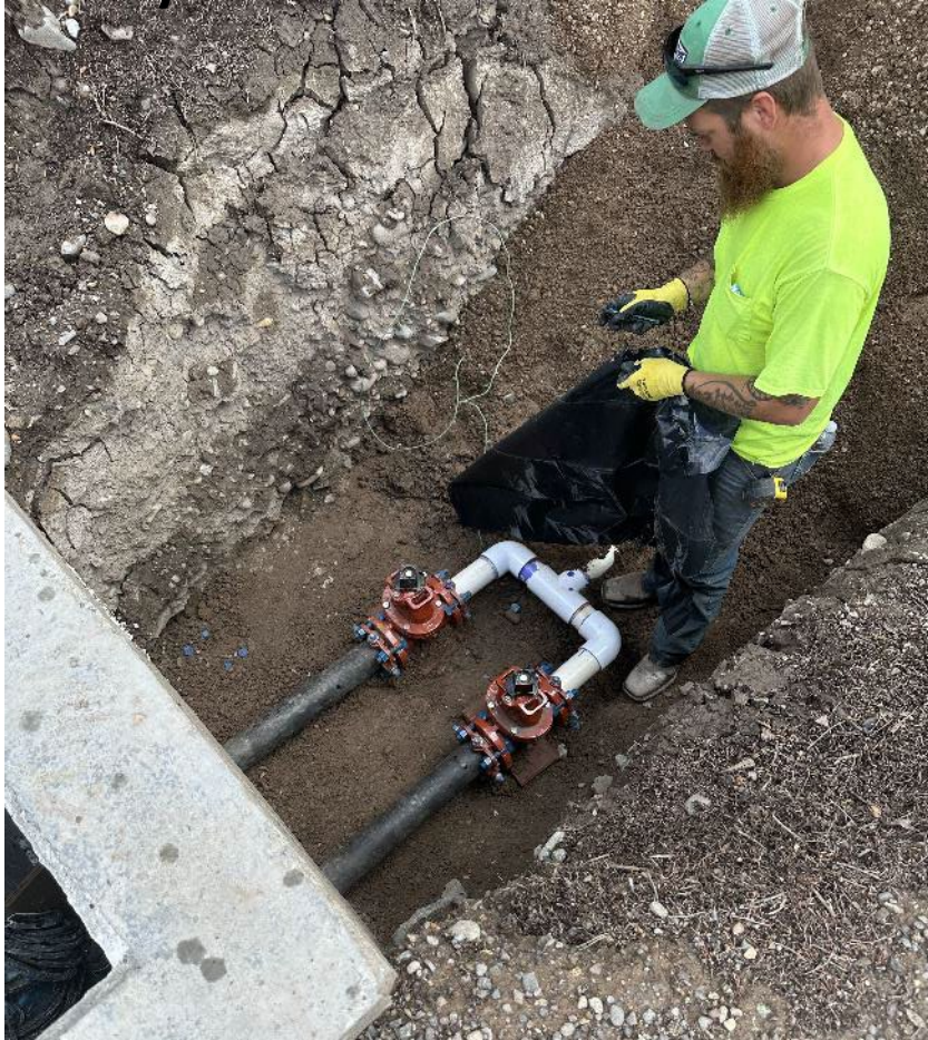
Piping outside the recycle vault
