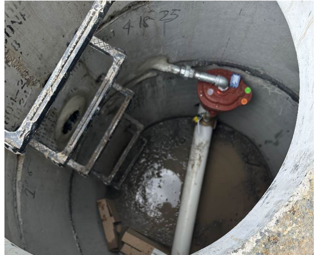
Air Vacuum Breaker for the recycle line
